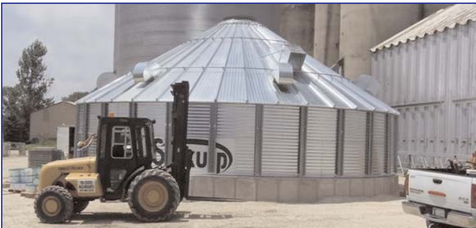
In this photo taken July 15th the bin crew had just finished adding the second ring to the new 100,000 bushel grain bin going up in Springville, with 22 more rings left to go before they were done.
